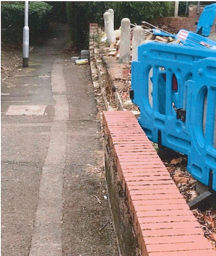
Original photo before the location was tidied, showing the damaged/missing section of wall. The section of wall that can be seen in the forefront is leaning, so would need to be removed as part of the rebuild.
